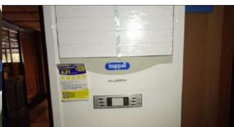
FLOOR STANDING AIR CONDITIONER (4 UNITS)
